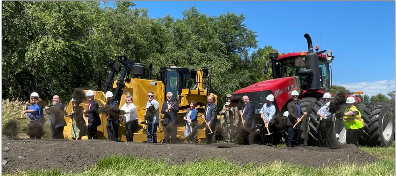
Corps senior leaders and elected officials shovel dirt at the P3 groundbreaking in Fargo, North Dakota, Aug 9. USACE St. Paul District photo by Shannon Bauer.
