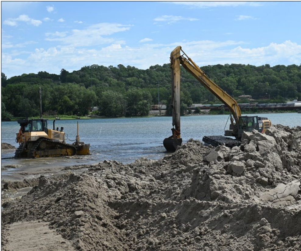
Construction operations at Pigs Eye Lake, near St. Paul, Minnesota, July 19. USACE St. Paul District photo by Melanie Peterson
